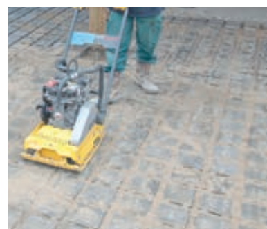
Photo 83 - Damage des joints.
